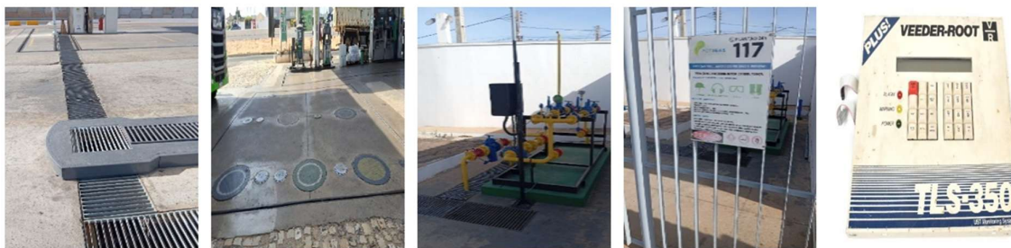
Figure 2. Monitoring Equipment, Systems, and Sensors. Source: Authors, 2026.
