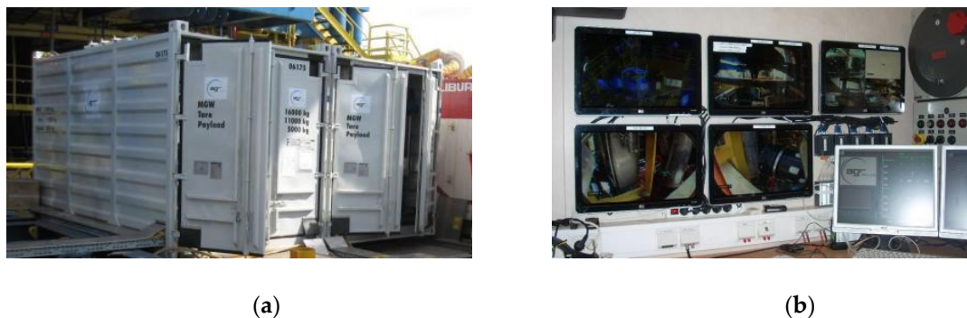
Figure 9. RMR control system [27]: (a) RMR control container; (b) RMR monitoring system.
