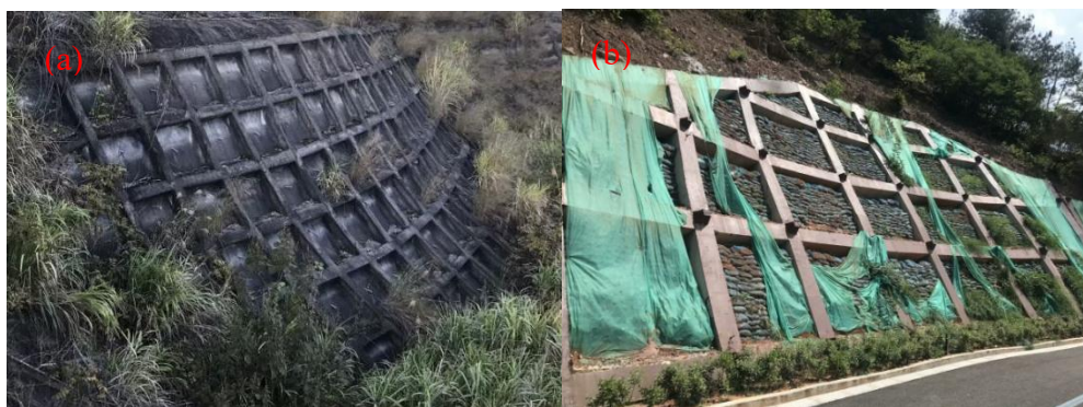
Figure 1. The frame beam slope anchoring system: (a) system with anchor bolts; (b) system with anchor cables.
