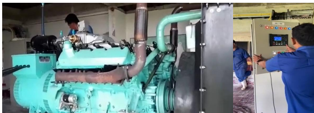
Figure 6. illustrates the operational testing of a diesel engine paired with a generator.
