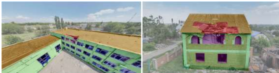
Figure 1. Examples of annotated images from our dataset (colors: Other - gray, Building - green, Roof - orange, Damage - purple, Damaged Roof - red, Broken Window - blue).
