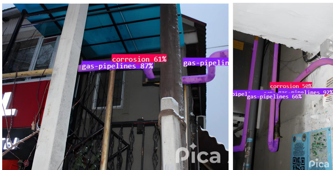
Figure 3. Example of corrosion detection and gas network element identification in a confined space using the trained models.
