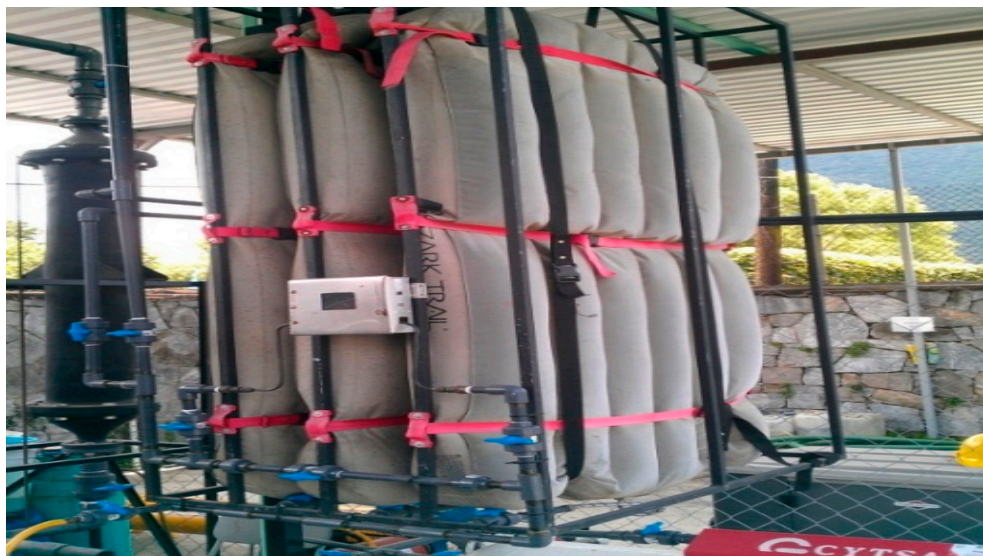
Figure 6. Biogas storage system.
