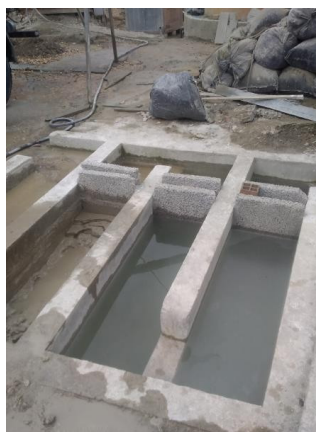
Figure 3. PTAR tanks. Source: Own.
