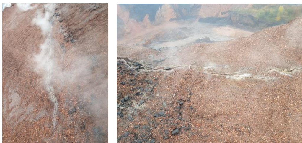
Figure 4. Occurrence of cracks/fractures on the slope surface caused by coal combustion within the dump body.
