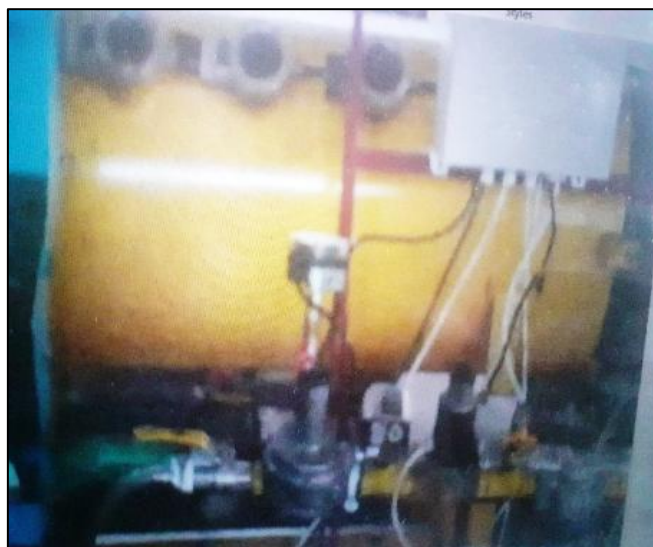
Figure 2. Partial image of the burner testing stand.
