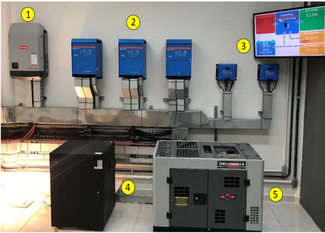
Figure 7. LAM Microgrid – Physical connection of equipment.
