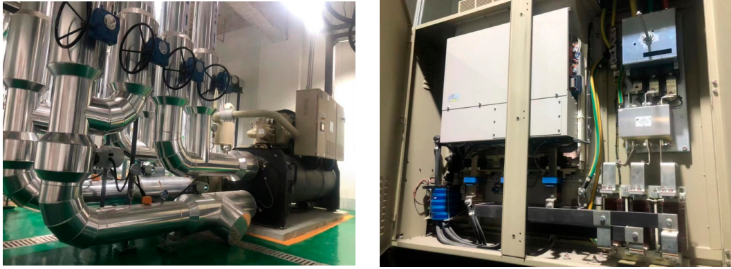
Figure 2. The heat-pump heating retrofit project located in Shanxi, China.
