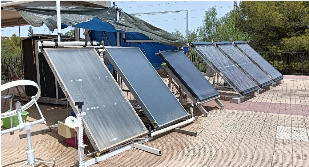
Figure 1. Solar collectors at the Solar Laboratory of the UMU. Conventional solar thermal collectors (left), PVT hybrid collector (centre) and vacuum tubes (right).
