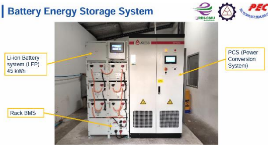
Figure 3. The figure (a) shows a 45 kWh Li-ion (LFP) battery energy storage system with a Power Conversion System (PCS) and Rack BMS.
