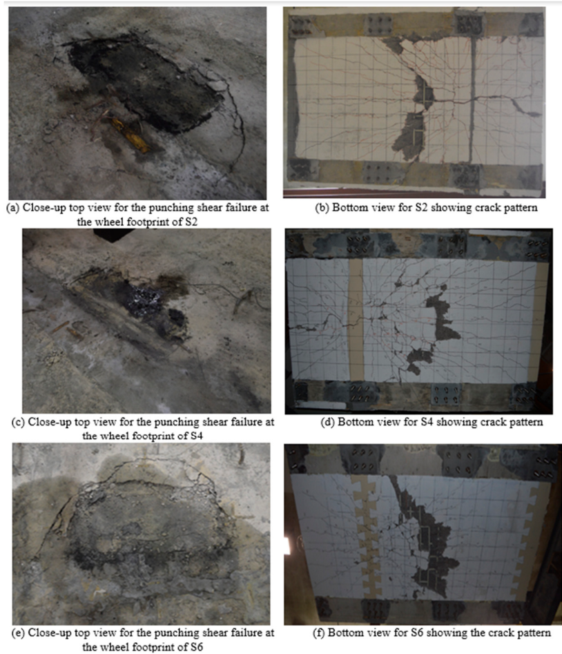
Figure 11. Views of punching shear failure of slabs S2, S4 and S6 tested under VAF loading to collapse.
