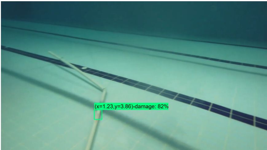
Figure 11. Location 1 of pipe line damage detection
