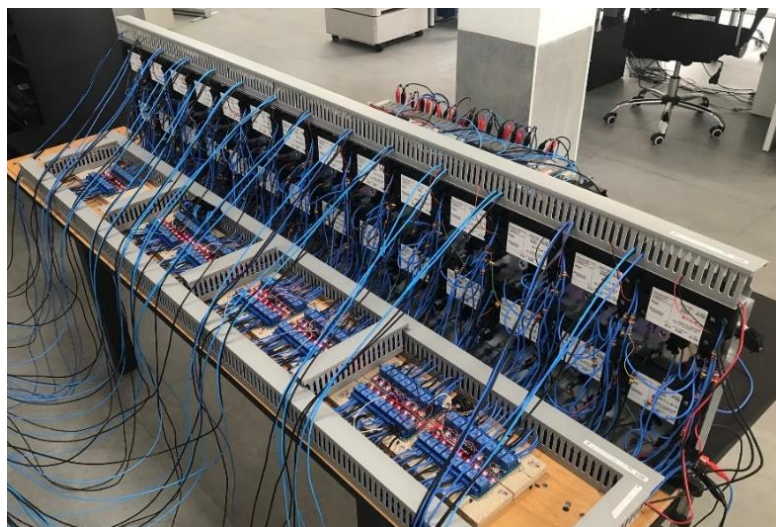
Figure 11. Rear panel with relays. Example.
