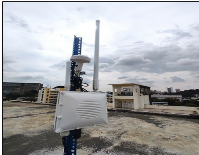
Figure 6. LoRa Gateway Positioned on the Rooftop.
