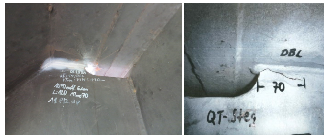
Figure 1. Crack between cover plate and cross member
