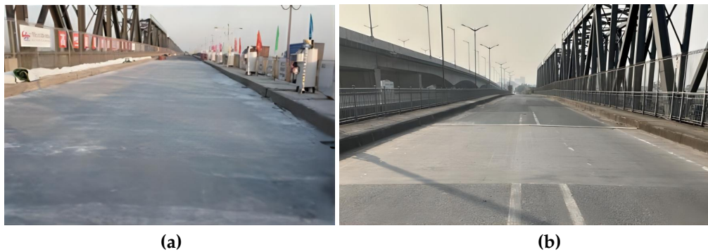
Figure 8. Mafang Bridge using steel-UHPC composite deck: (a) Under construction; (b) After 12 years in service.
