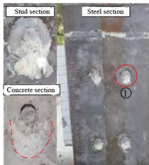
Figure 11. Photo of stud shear failure.
