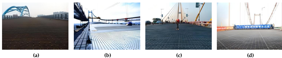
Figure 9. Bridge deck under construction: (a) Fochan New Bridge; (b) Hangrui Dongting Lake Bridge;(c) Queshi Bridge;(d) Fengxi Bridge.
