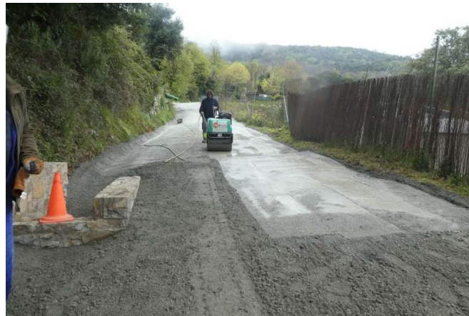
Figure 15. Rainwater harvesting by paving roads and rainwater collection ditches.
