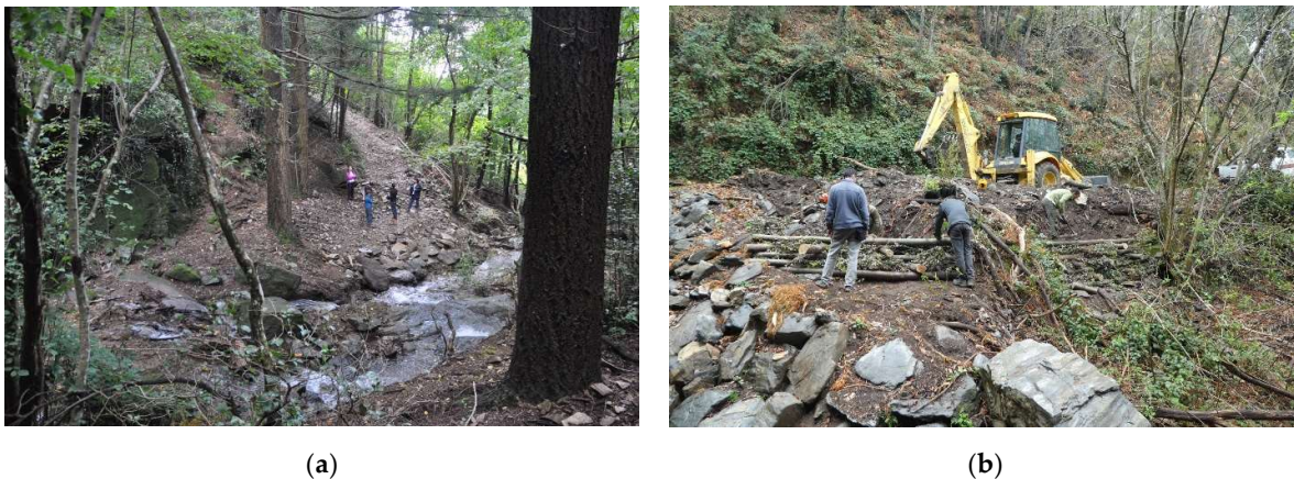
Figure 16. Restoration of the autochthonous forest placed in the secondary basins where the species lives using bioengineering techniques and traditional materials from the forest. The kind of installed structures varies according to the characteristics of the slope and the length of the affected section. (a): before restoration. (b): during restoration.
