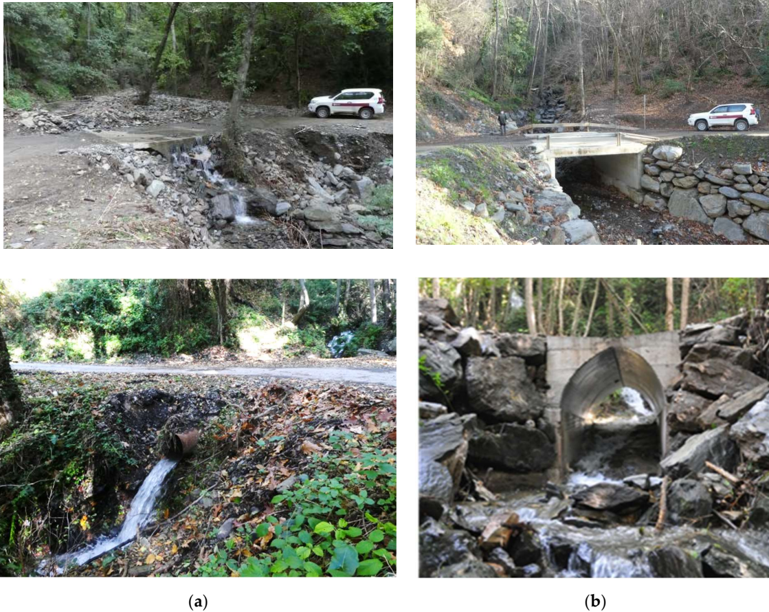
Figure 17. Modified bridges to recover the natural stream bed and to allow the displacement of aquatic fauna along them. (a) images: before recovering structure. (b) images: after recovering structure.
