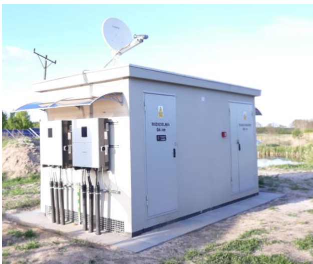
Fig. 6: Satellite Antenna mounted on the top of the transformer station
