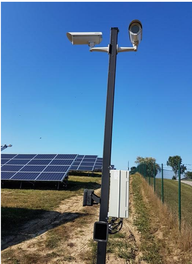
Fig.8: Uniview camera and lamp mounted over a pole for CCTV surveillance, I+D Energías, Poland
