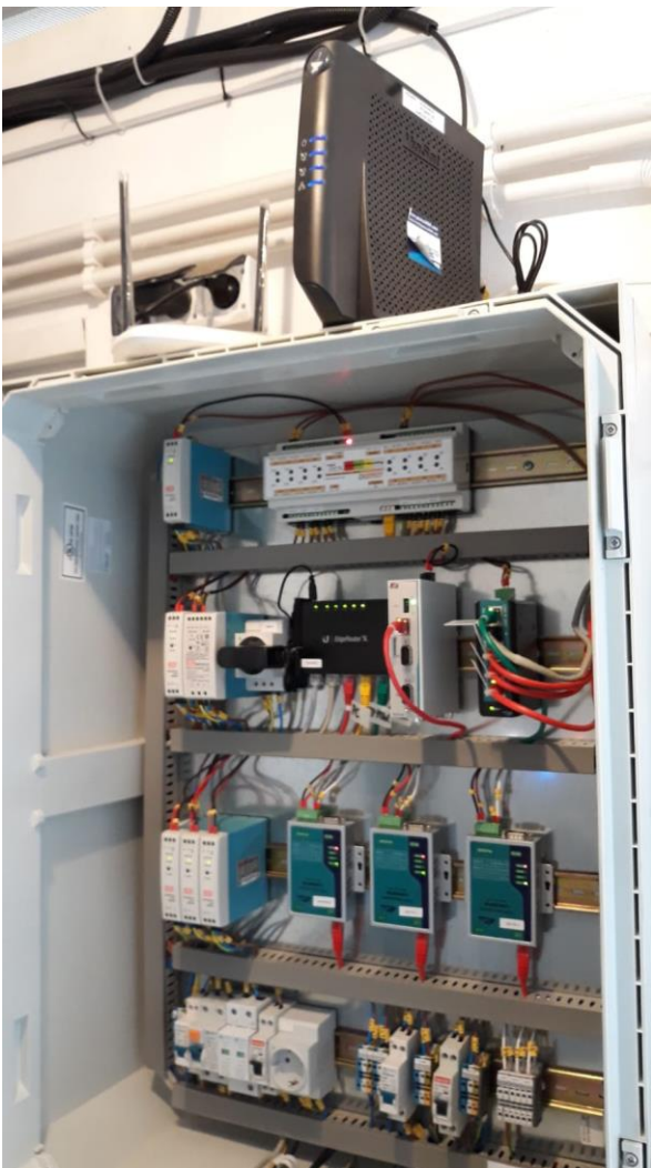
Fig.5: Satellite Modem and Router already connected to the monitoring cabinet, inside transformer station.
