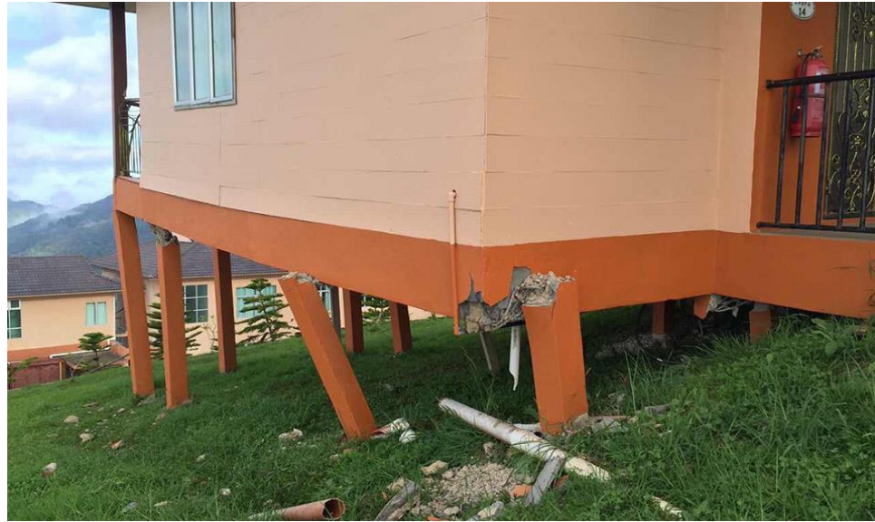
Figure 6: Cracks on room pillar of Dreaan World Resort Kundasang
