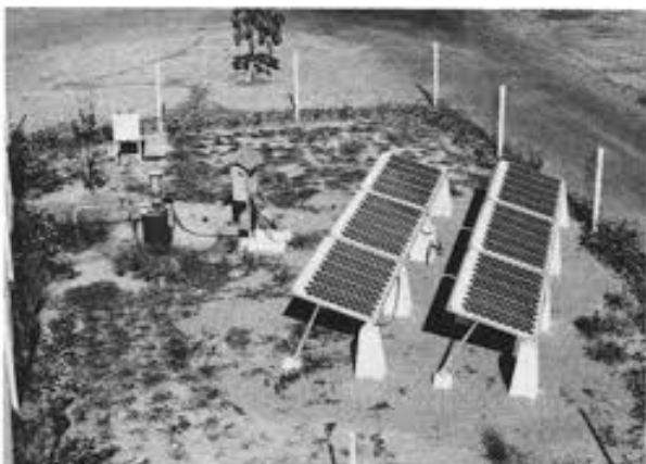
Figure 1. One of the first photovoltaic pumps installed in Mali by Father Verspieren’s community. The three PV modules reached a 900 W peak power. [Reproduced from Ref.11].
