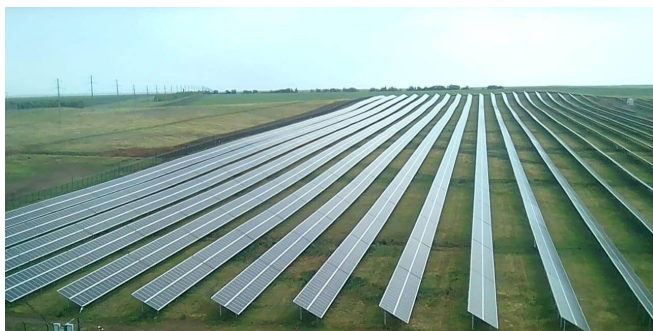
Figure 1. The Yelshanskaya 25 MW photovoltaic park in the Orenburg region supplies power to the grid since July 1, 2019. Using only components made in Russia, the plant is expected to produce 30.5 million kWh annually. [Image courtesy of Hevel Energy Group, Reproduced from hevelsolar.com].
