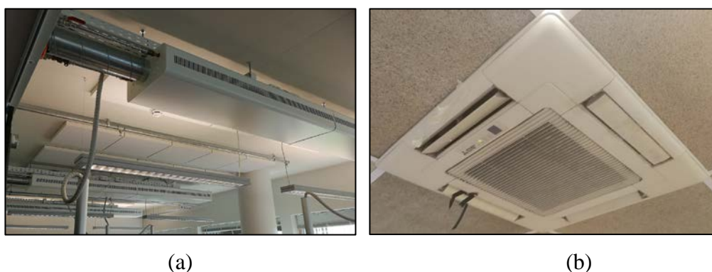
Figure 2. (a) Possible air flow obstacles with open active beam solution; (b) Modified airflow distribution with fan coil unit.
