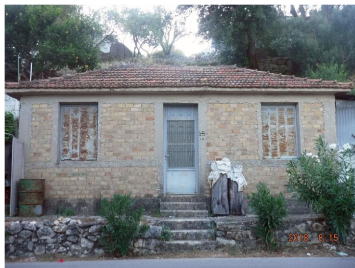
Figure 7. Confined masonry one-storey house in Pastra, with fired-clay bricks, in present condition.
