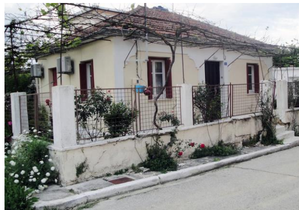
Figure 5. One-storey arogi house in Lixouri after the 2014 earthquake.
