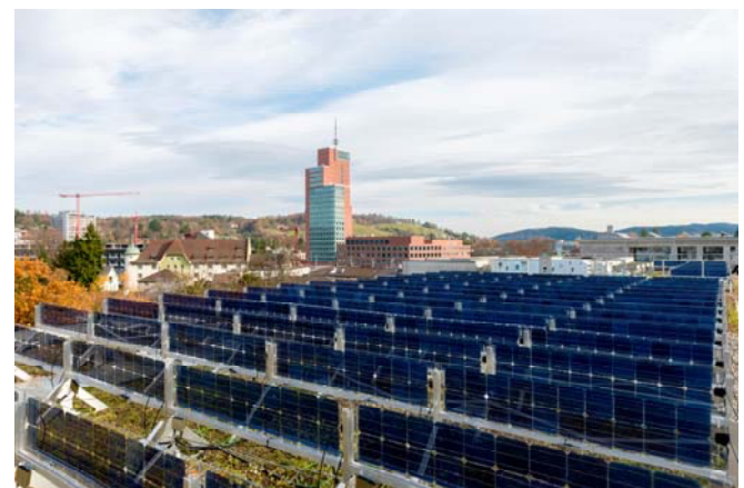
Figure 5. Aerial (top) and later (bottom) view of the 9.09 kW photovoltaic array on the rooftop of a building of Zurich University of Applied Sciences in Winterthur. [Photo courtesy of T. Baumann and Zurich University of Applied Sciences].
