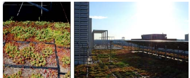
Figure 2. Effects of protection from the PV array on the green roof where vegetation appears to have greater coverage ( left ) in areas shaded from direct sunlight for a portion of each day ( right ). [Reproduced from Ref.17, with kind permission].
