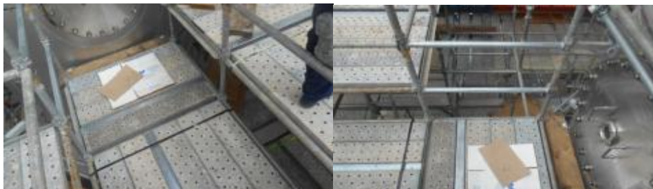
Figure 4: Work Area with Visible Gaps
