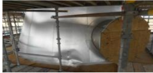
Figure 5: Damage to Brine Concentrator – Post-Impact
