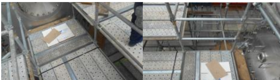
Figure 4: Work Area with Visible Gaps
