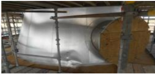
Figure 5: Damage to Brine Concentrator – Post-Impact
