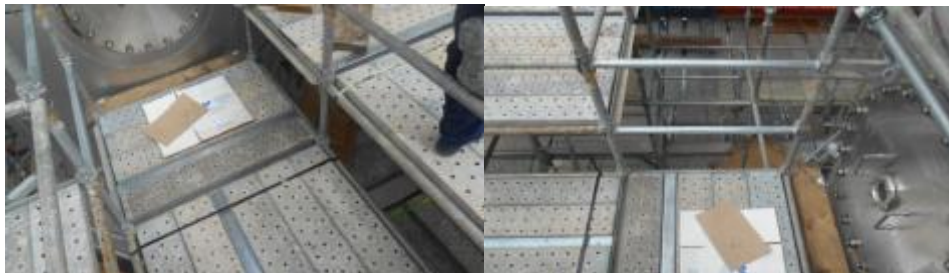
Figure 4: Work Area with Visible Gaps
