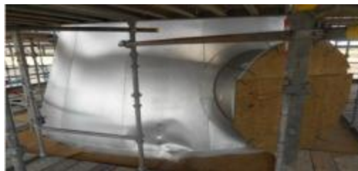
Figure 5: Damage to Brine Concentrator – Post-Impact
