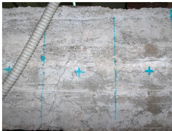
Figure 8: Cracks at the incoming collapse
