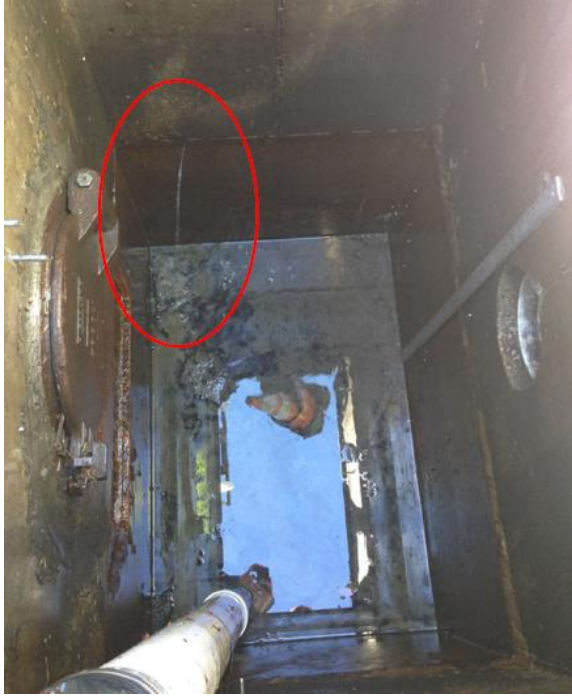
Figure 6. Leaking point in the inlet structure (Date: January 25, 2017)
