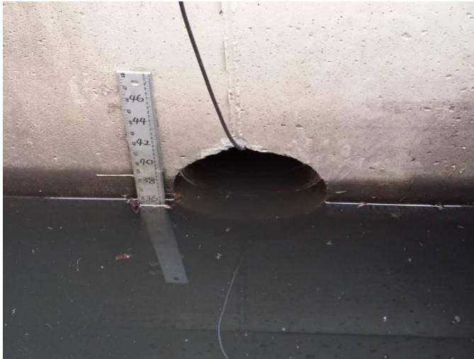
Figure 3. Ponding in the inlet structure due to partial clogging of the distribution pipe (Date: March 30, 2017)
