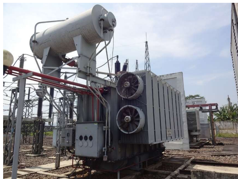
Figure 1. A sample of 150 kV power transformer used in this study
