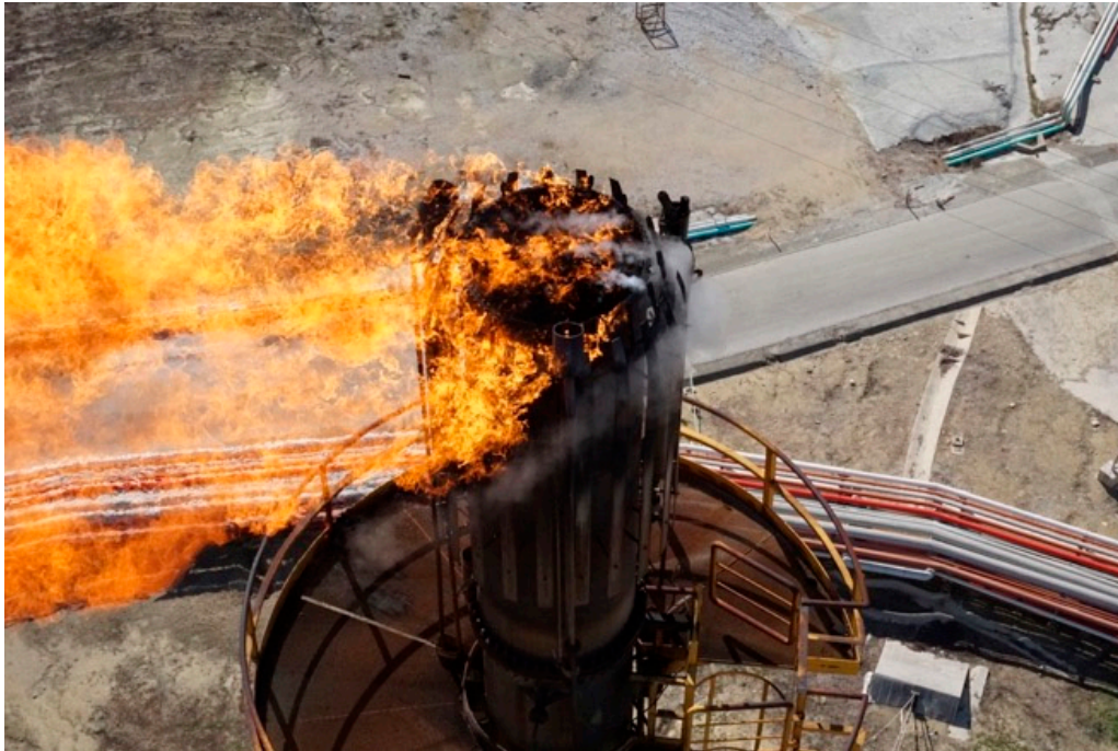
PHOTO 9. Image from above the burner area (tip) of a flare stack with a defect in the steam seal using a drone
