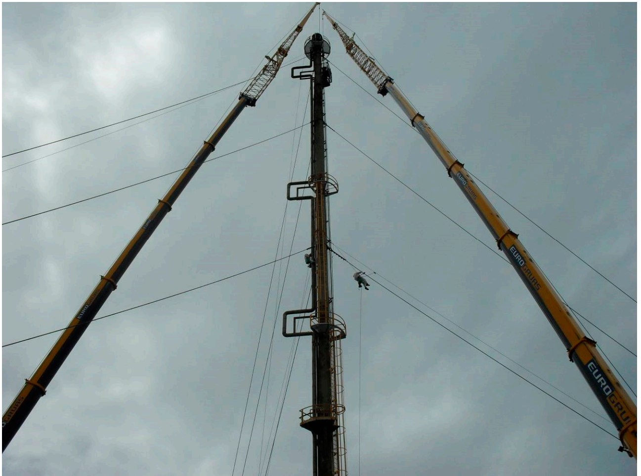
Fig. 02 Works on a flare stack using cranes and baskets, combined with rope access techniques for the inspection and lubrication of guy wires
