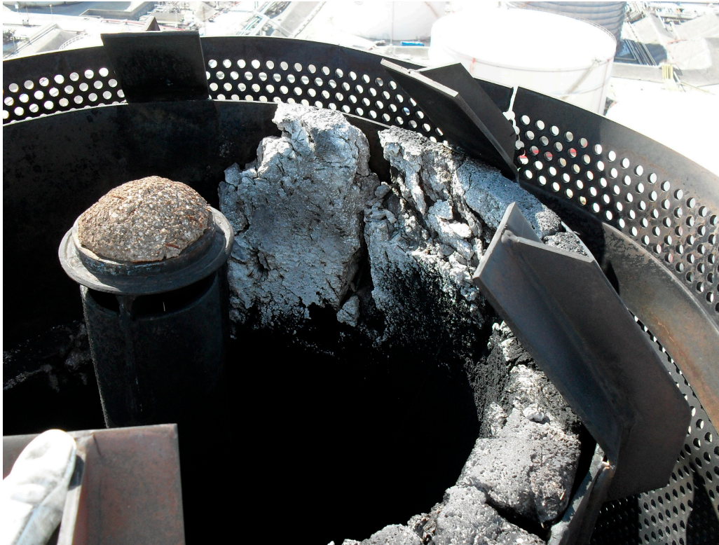
PHOTO 8.1 View from above of an installed burner, with detachment of fireproof coating
