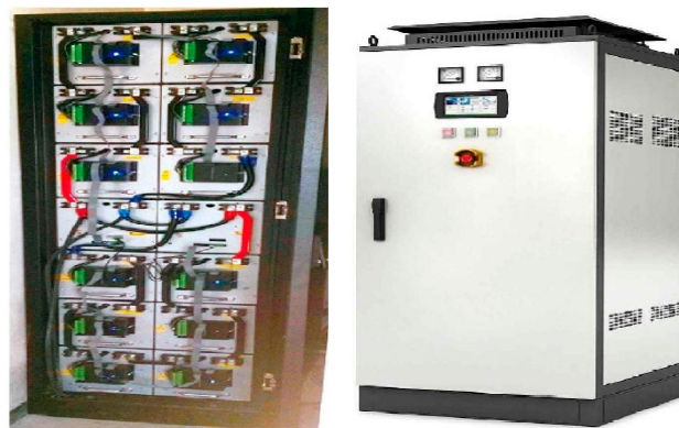
Figure 3. Battery (left) and PCS (right) on rooftop
