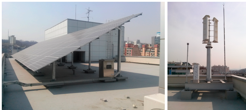
110 Figure 2. PV and WT system at Guri Office
