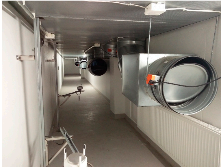
135 Figure 4. Supply air duct corridor and classroom-specific ducts' terminal units. Dampers are opened 136 20%, as designed.
