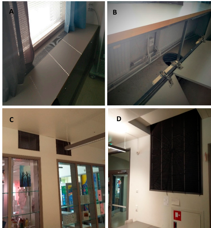
116 Figure 3. (A and B) Supply air grill and duct in the classrooms, (C) transfer air grilles in the 117 partitions between classrooms and the lobby, and (D) exhaust stack in the lobby.
