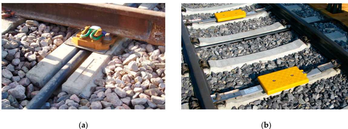
Figure 2. Needs for modification to suit cables and pipes (a); and advanced signaling systems (b).
