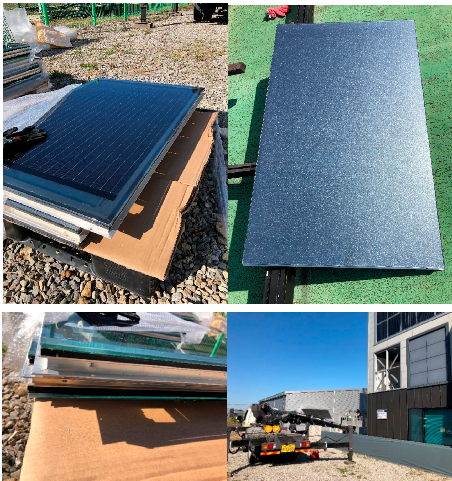
Figure 6. Conventional and gray-colored modules tested on the Mock-up building.
