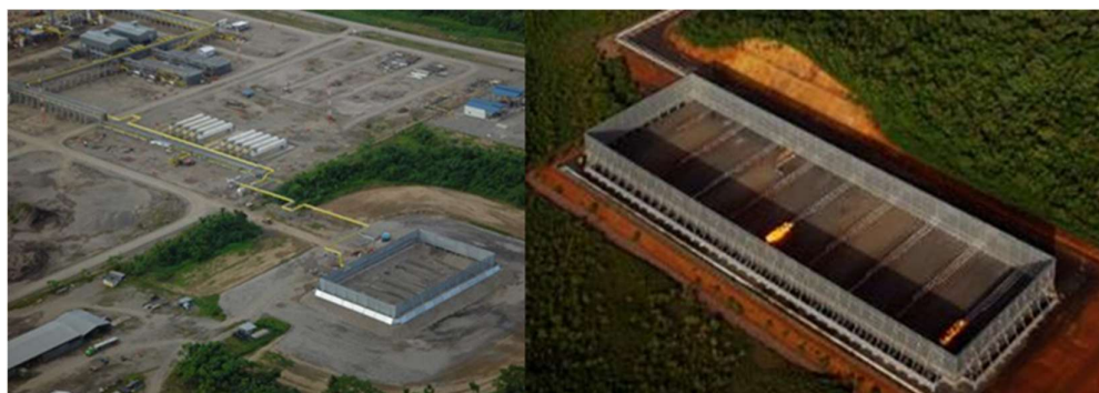
Figure 3. Multi-Point Ground flares built and operated as part of a petroleum production (courtesy Zeeco, Inc.).
