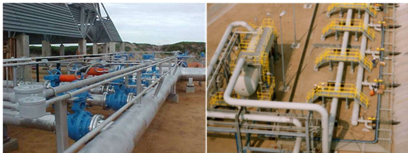
Figure 5. Modern ground flare system includes complex piping systems to stage flare gas to accommodate wider operating ranges with high combustion efficiency (courtesy Zeeco, Inc.) [2].
