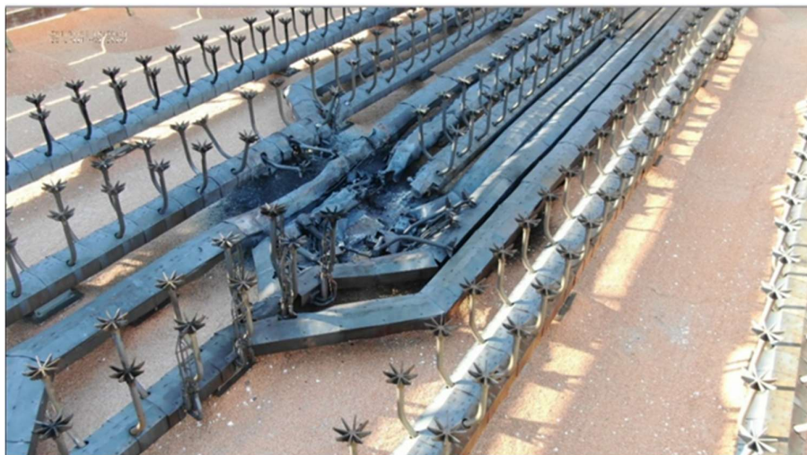
Figure 16. Heat damage to MPGF runners (courtesy Zeeco, Inc.).
