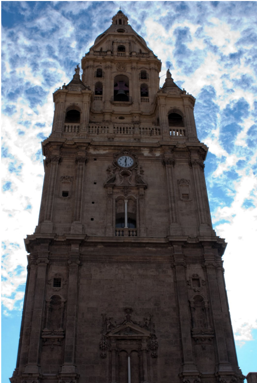
Figure 8. Northern elevation of the tower showing the second and third tiers, conjuratorios, and bell chamber. The successive deviations from verticality and compensations applied during construction are visible (photograph by the author).
