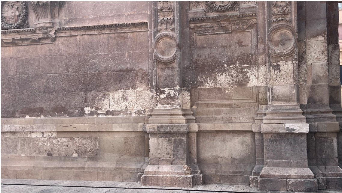
Figure 7. Sound and deteriorated limestone at the base of the tower, east façade (photograph by the author).
