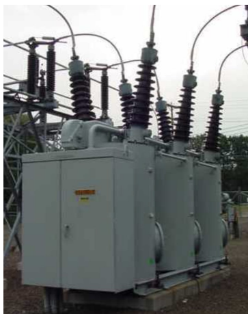
(a) Physical installation of a high-voltage circuit breaker in an outdoor substation.
