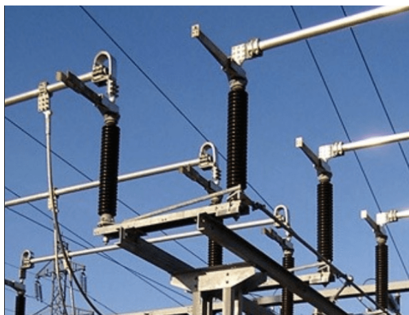
Figure 10. An open disconnector showing the visible isolation gap. Adapted from [57].
