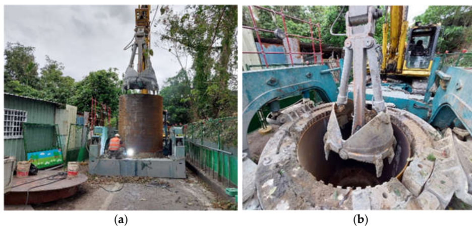
Figure 2. On-site photographs of key construction machinery and equipment deployed at the Hualien project site. (a) Casing Oscillator; (b) Tubular steel casing.
