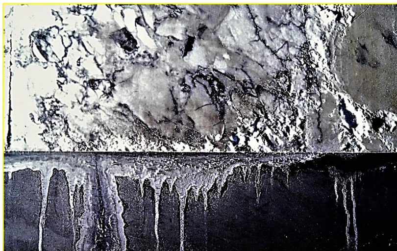
Figure 6. Santa Maria dei Miracoli Church. On the lower part salt efflorescence are visible; on the upper part sub-efflorescence are detaching small flakes of marble.
