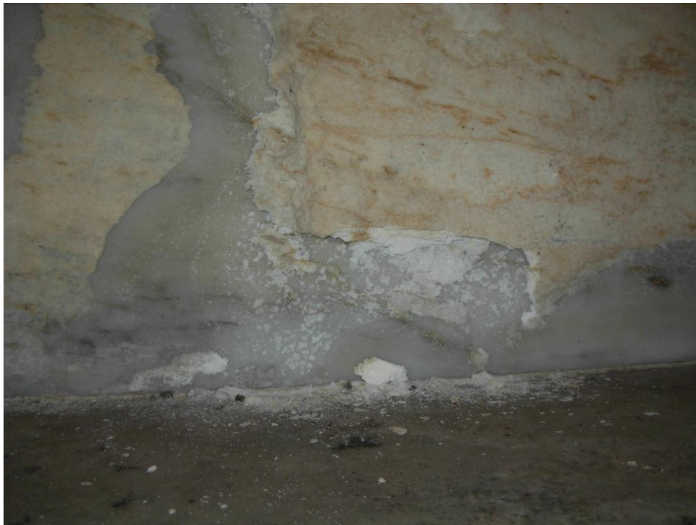
Figure 11. Exfoliation of thin marble layers due to salt crystallization at sub-surface level.
