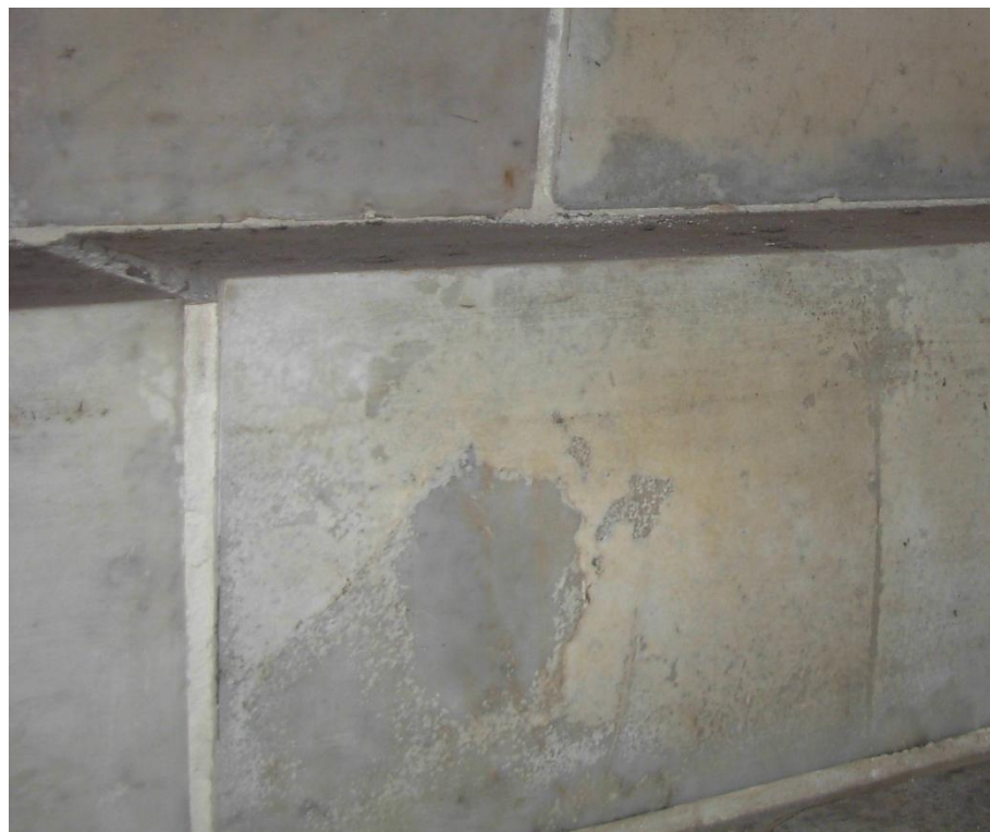
Figure 10. Whitish surface areas, slightly eroded. The explanation of this feature is discussed by optical and SEM microscope analyses. The pale yellowing areas are ascribed to iron oxides formation due to oxidation of small particle of pyrite ( \text{FeS}_2 ). The yellowing is a natural weathering alteration due to the presence of this small iron impurities in the Carrara marble.
