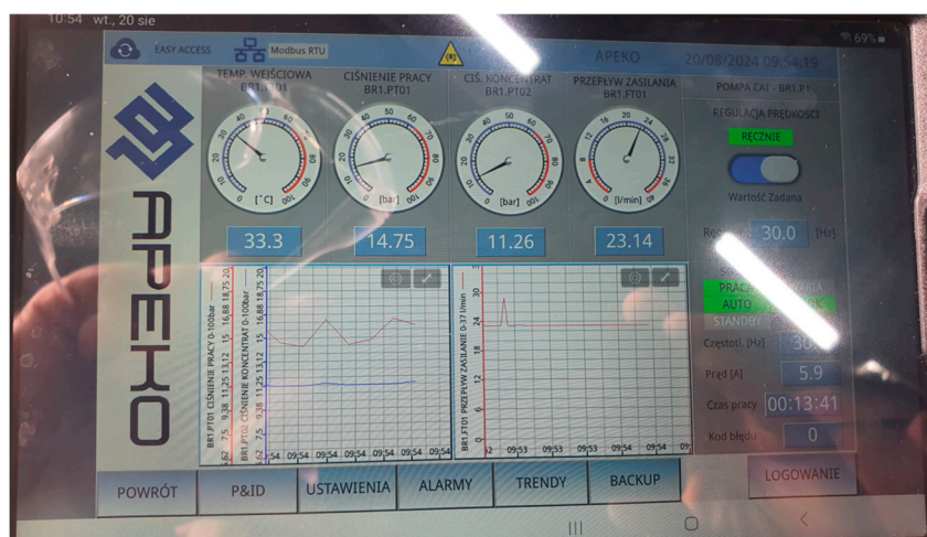
Figure 3. Screen of the APEKO UF – 1 pilot installation controller (own photo).
