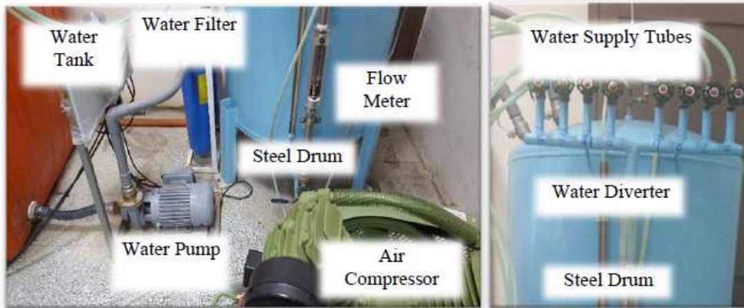
Figure 6. Front-End of the Water Supply System.
