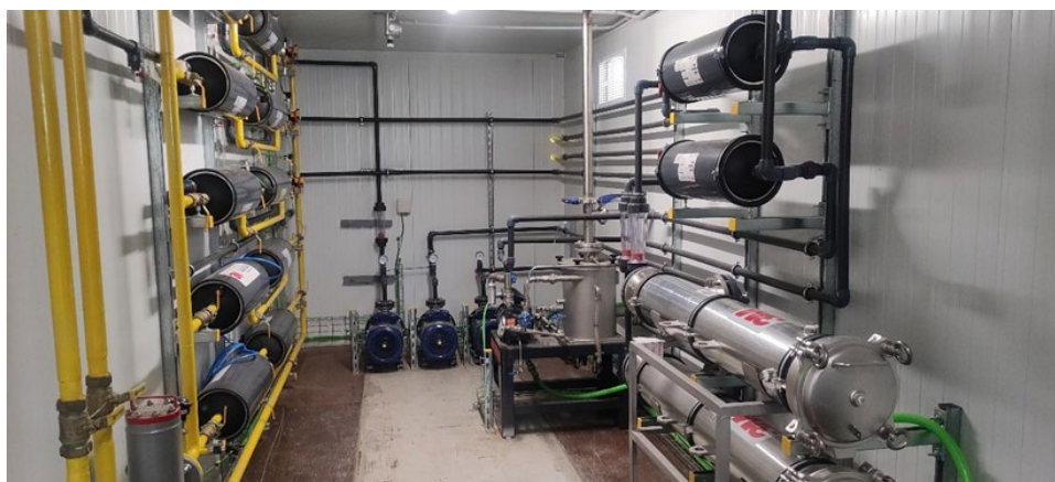
Figure 7. Membrane contactor system for biogas upgrading (Spain).
