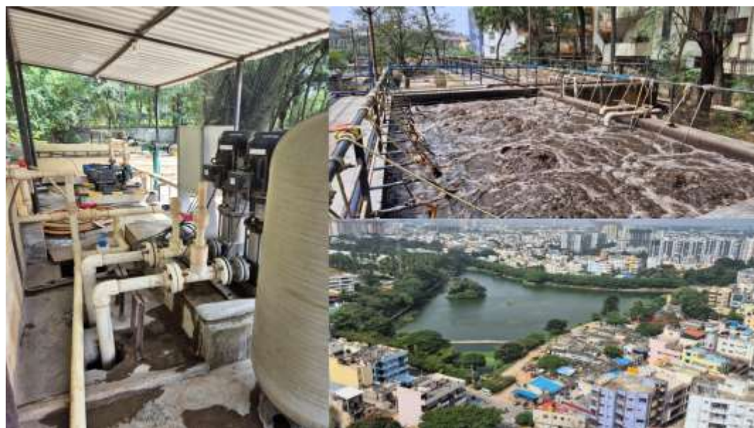
Figure 3. Photographs taken during fieldwork in South City. The images illustrate key components of the local wastewater management system that supports both residential water reuse and lake restoration. Left: filtration and pumping infrastructure distributing treated wastewater for non-potable use within the residential complex or discharge toward the nearby lake. Top right: aeration tanks at the decentralised sewage treatment plant (STP),
