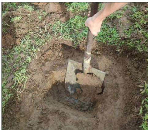
Figure A.1.2. Scraping and Trenching to access the upper layer of prospected clay deposit.
