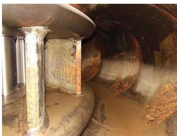
Figure 3. Corrosion/erosion to the spiral casing and stay vanes.
