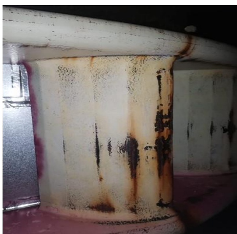
Figure 1. A damaged stay vane.
