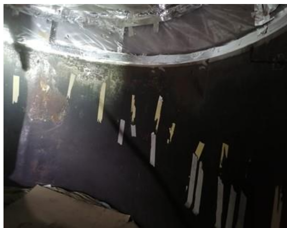
Figure 2. A damaged cover.
