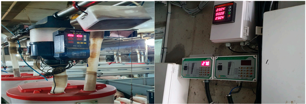
Figure 6. Photos of the RS485 and MQTT equipment installed in Suncheon City.
