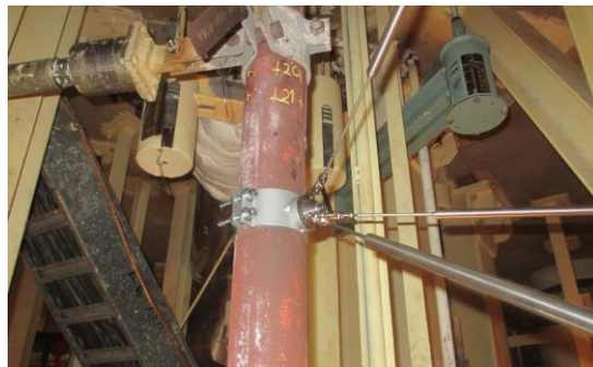
Figure 8. Mounting of the inductive displacement transducers on the pipe at the observation point S.
